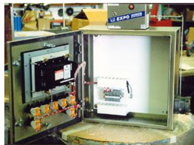
(Purged Panelview Enclosure)
